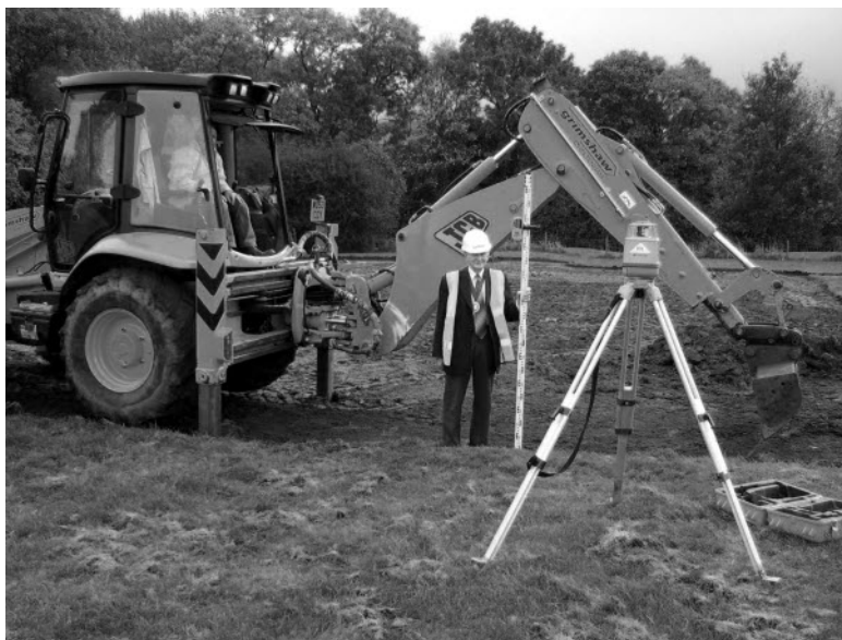
David Folkes, Chairman of Broadway Parish Council using a laser and levelling staff, assisting the JCB driver to excavate for the MUGA's area of the new Activity Park on the 15th October.
