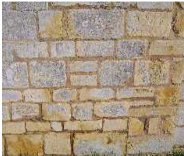
Illustration 24: Poorly maintained walls
