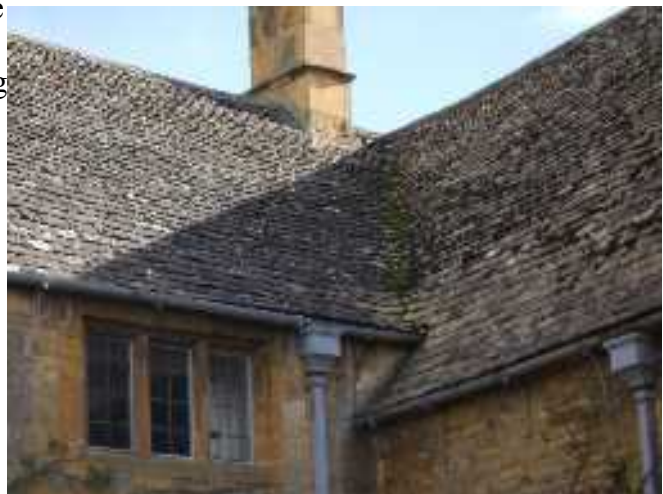
Illustration 32: The construction of swept valleys is the best example of this skill. Cut slates were used to form a gently curve to the roof through 90 degrees. The slates used 2 across the valley, alternating with 3 across and where there were 3, the centre slate was wedge shaped and did not require a peg.
